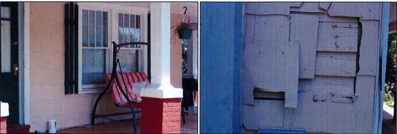
Figure 24. Wall House: west front elevation with Craftsman-style porch, sash, and front door at left; north side elevation with original German siding exposed beneath asbestos shingles at right
